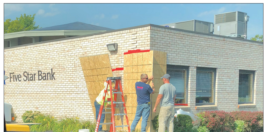
Workers board up the area where a vehicle crashed into the Five Star Bank building on Friday. Photo by Donna MacKenzie
